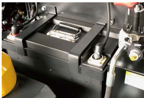
24V/80Ah Lithium battery has connection terminals with screws and is protected inside the steel case.
