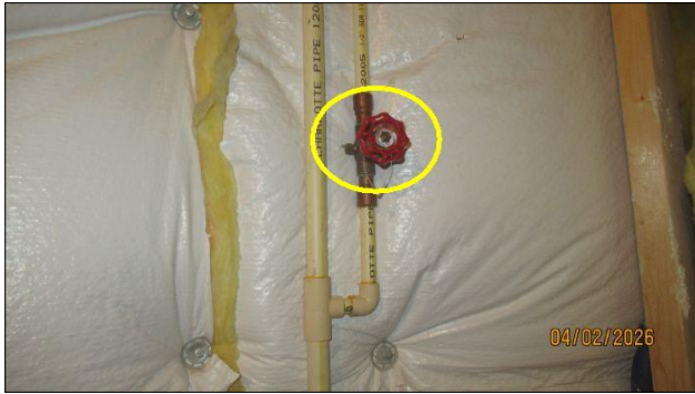
front hose bib shutoff
