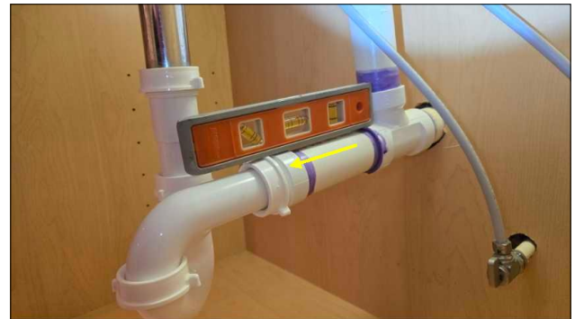
drain slopes forward
