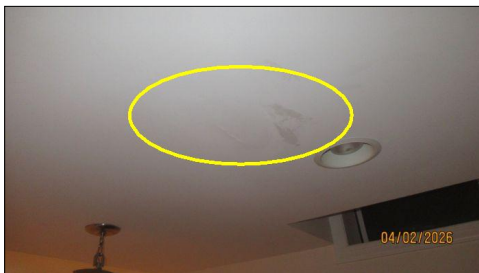
basement bar ceiling leak
