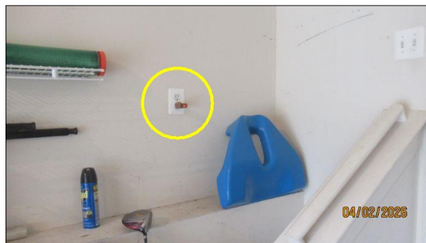
outlet not GFCI protected
