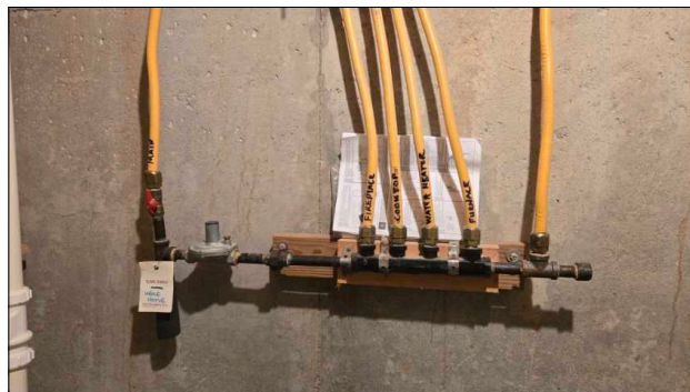
No visible bonding
