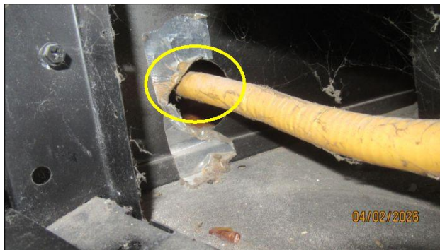
no sleeve for gas line
