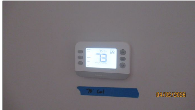
main level t-stat loose
