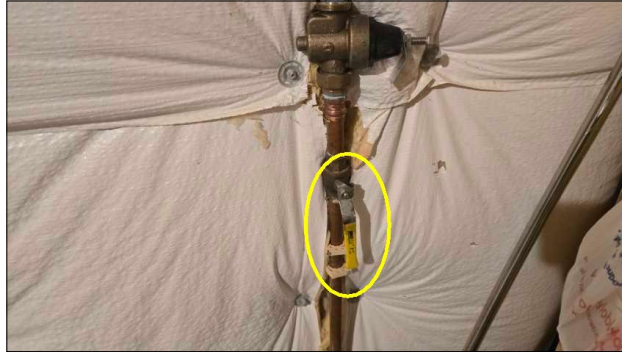
Main water shutoff valve
