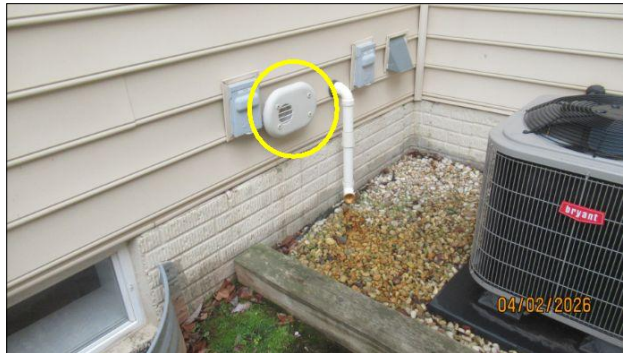
furnace flue exhaust and intake
