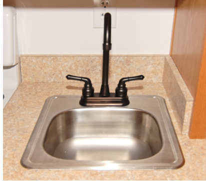
Wet Bar Sink
