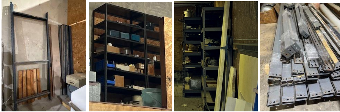
Steel rack systems collapsing=2
