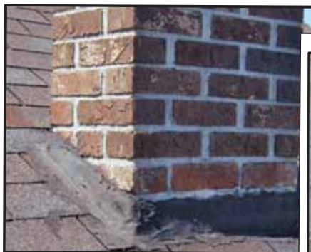
Chimney with cracked and deteriorated flashing
