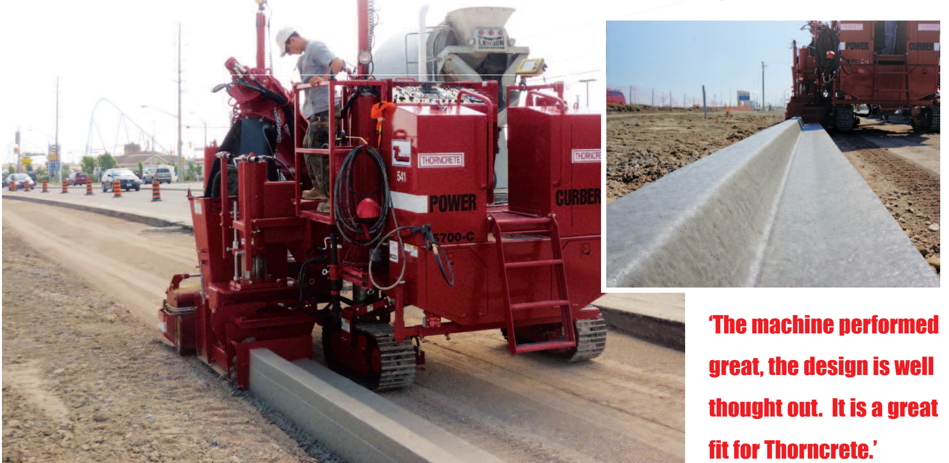
Above: 5700-C, with Topcon Millimeter GPS controls, pouring without stringline in Toronto. Inset: Smooth and straight, and no stringline to set and take down.
