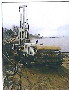
Soil Sampling This 7822DT collects DT22 (dual tube) samples along a damaged sea wall. Because of its lightweight and compact size, the rig was able to drive along the beach without the use of tracking pads.
