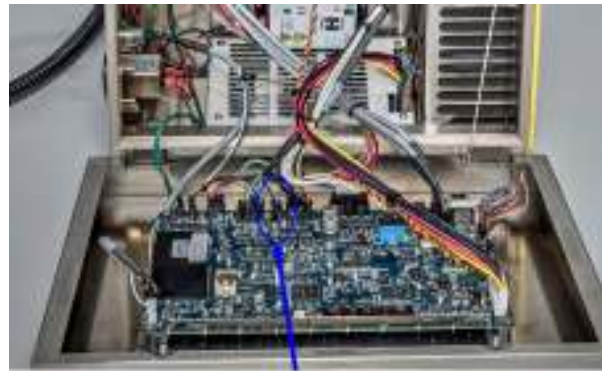
Pressure Transducer cable connection at J13
