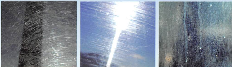
Examples of unprotected, scratched, stained and encrusted glass.
