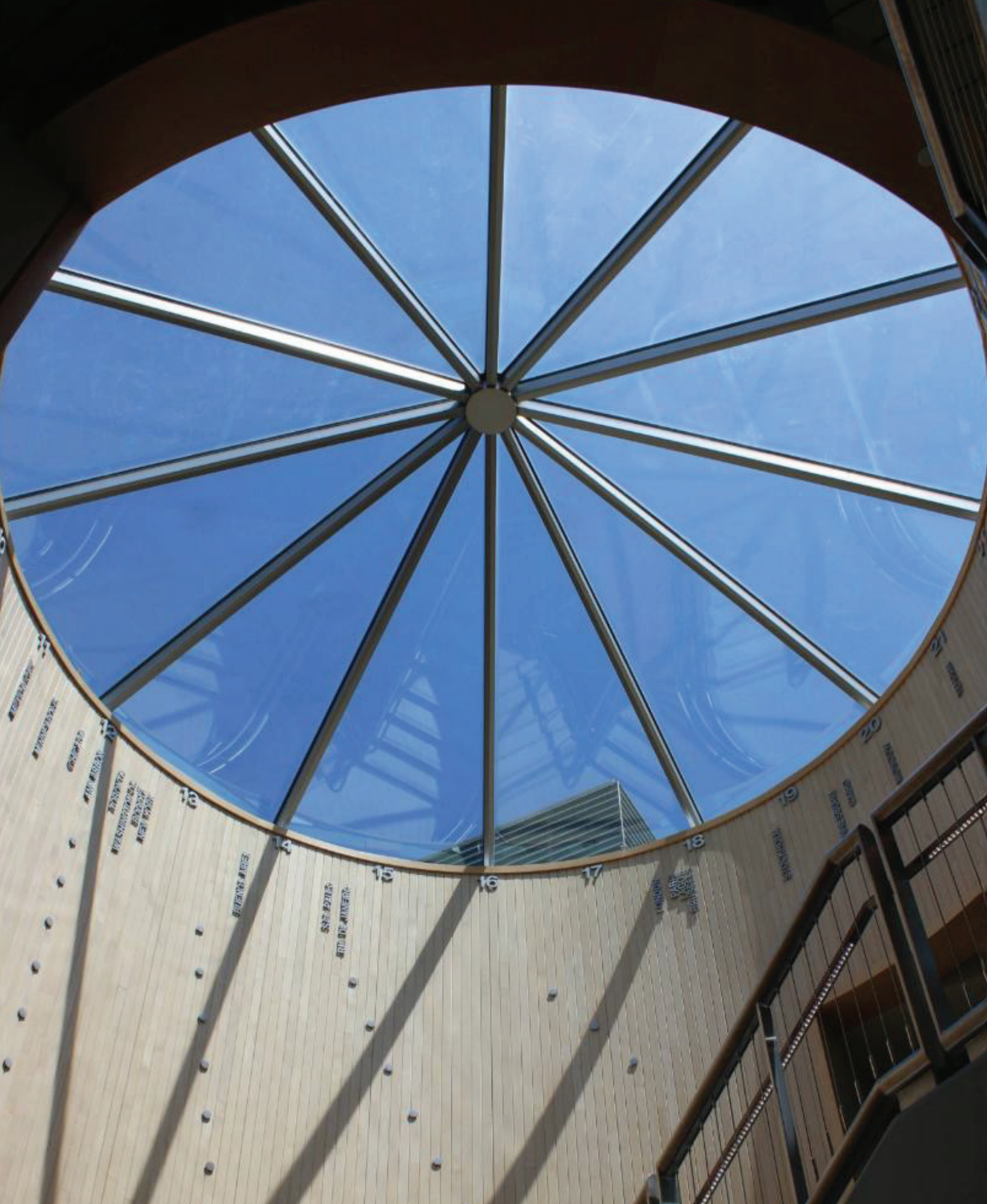
University of Michigan, Memorial Phoenix Lab - Ann Arbor, MI Architect: Lord Aeck Sargent Architecture
