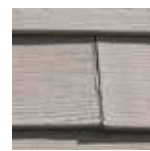
FIBER CEMENT Cracking, Fading, Off-Gassing
