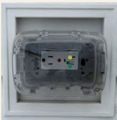
Exterior GFCI Receptacle
